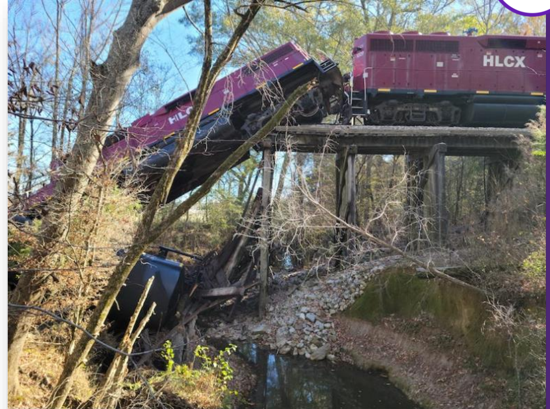
One locomotive and multiple cars derailed when a Grenada Railroad bridge collapsed on Wednesday. Photo by Debbie Fly Hayward via Facebook.
